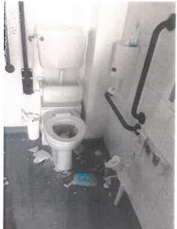
Photo 4 All WCs smashed, human waste left.
