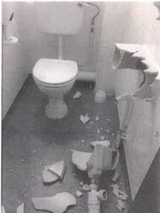
Photo 3 All WCs smashed, human waste left.
