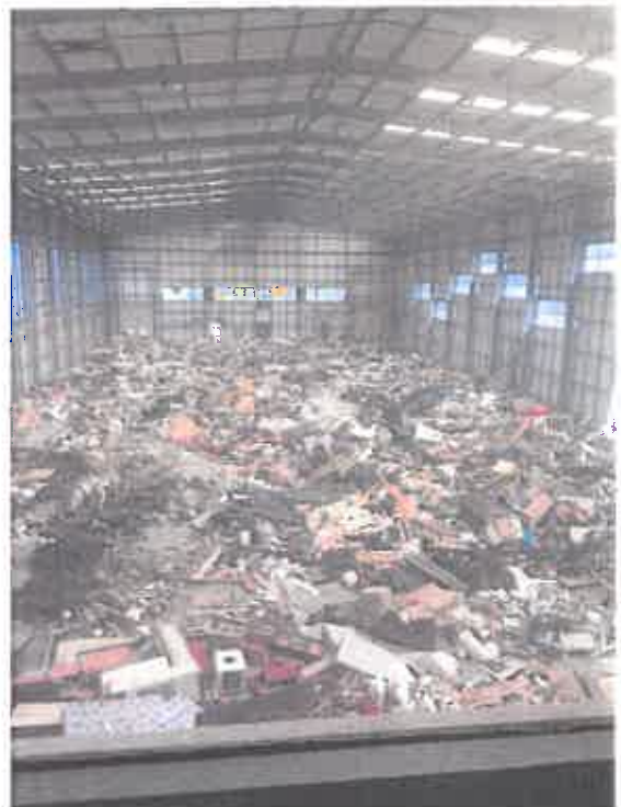
Photo 10 Waste tipped internally.
