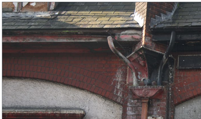
Broken gutters prevent water flowing away from a building.
