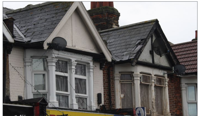
Slipped and missing tiles need to be replaced to prevent water ingress and damage to the roof structure
