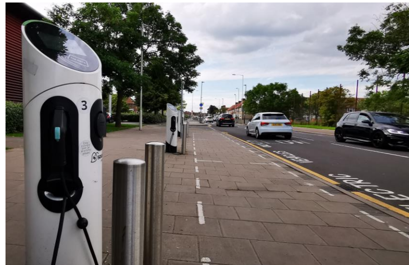
Figure 27 – On-street EV Charging Infrastructure
