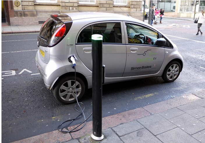
Figure 24 – Example of on-street EV Charging Column
