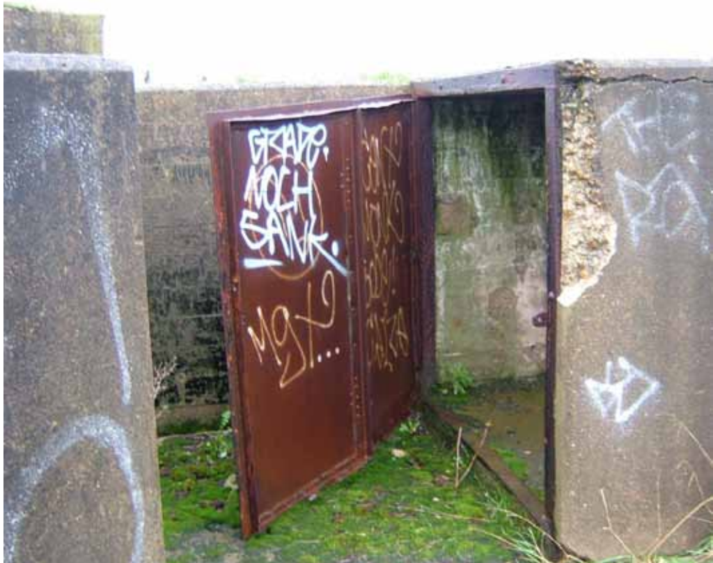
Figure 15 showing a close up of the concrete structures and metal fittings (source: the writer)
